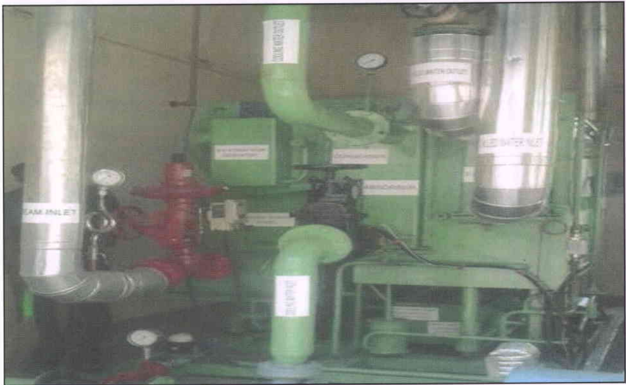
Vapour Absorption Refrigeration unit at Gokul Dairy, Kolhapur
